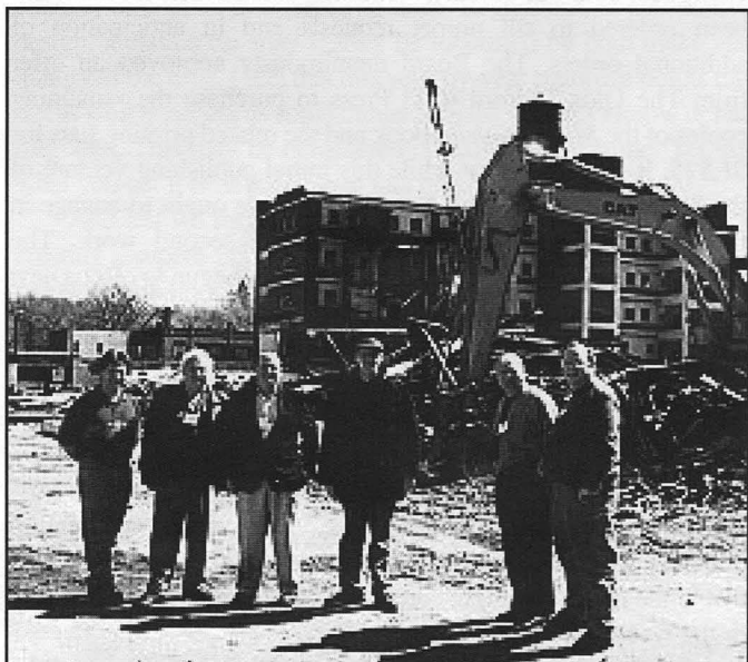
On a tour of Cleveland factory sites, the board members were on hand to watch the demolition of the former Stearns plant.
